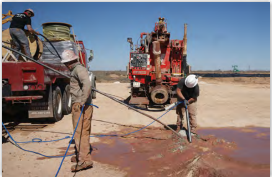
The Durammo™ Deep Anode System installed to protect oil wells in Texas from corrosion.
